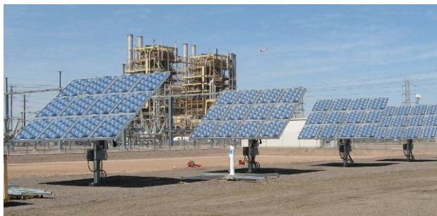
Figure 1. Four of the five SolFocus 2.5 kW arrays at the APS-STAR center in Tempe, AZ.
